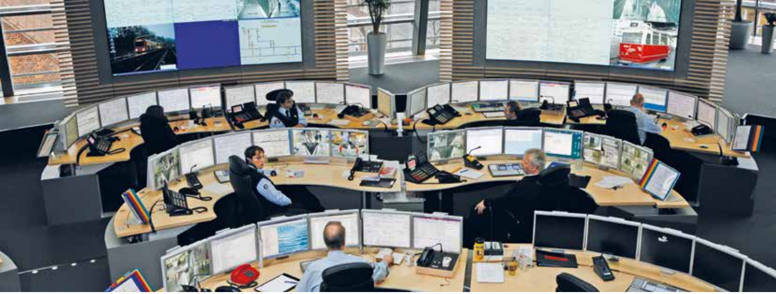
Subway control center of the Hamburger Hochbahn AG
