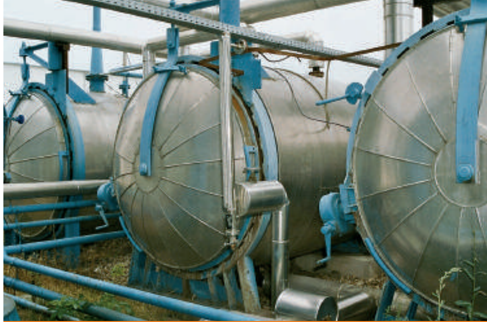
Autoclaves for steam-curing building materials
