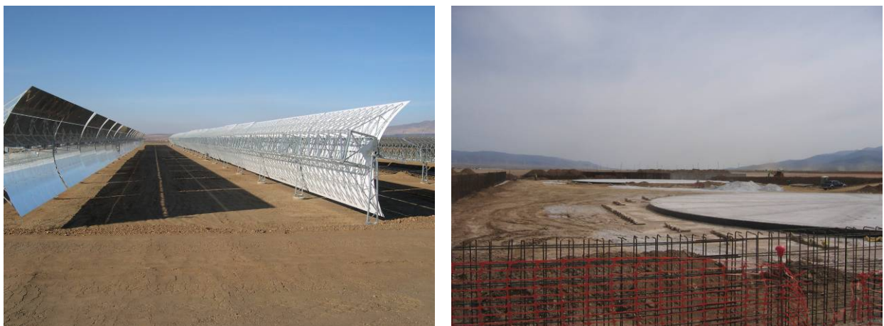
Figure 1-16: Parabolic trough collectors and foundations for the molten salt tanks of ANDASOL 1.
