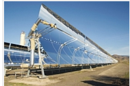
Parabolic trough collectors of the DISS-test facility for direct steam generation at Almeria, Spain
