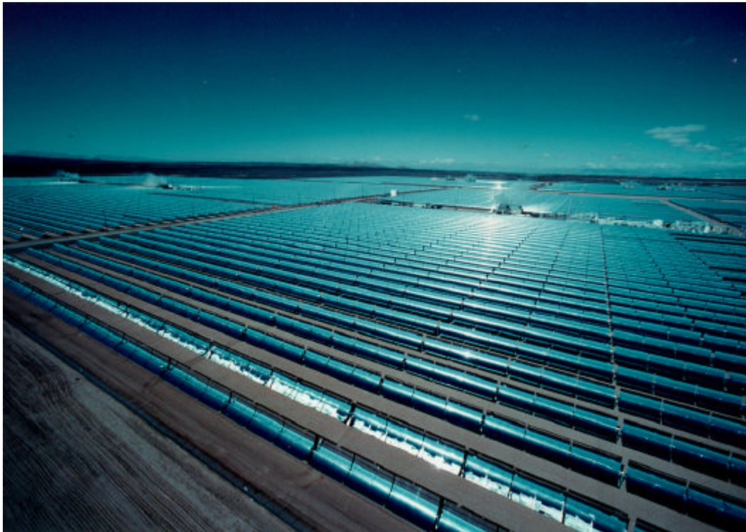
Fig. 1 Solar power plant of SEGS type in California (source: Pilkington Solar International)
