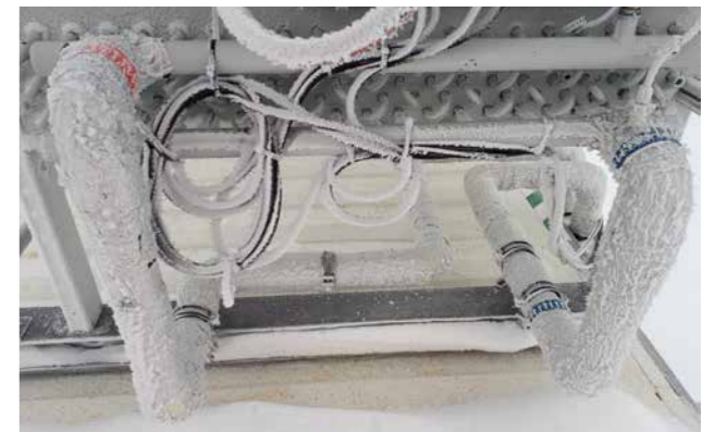
Frozen surface of the thermal control piping system on the roof of the EDEN ISS greenhouse
