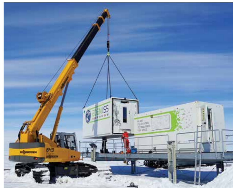
The EDEN ISS containers being installed on a raised platform near Neumayer III
