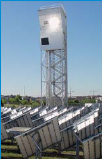
Solar plant SUN-to-LIQUID in Móstoles © ARTTIC / Christophe Ramage
