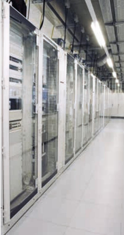
Large server farms in Neustrelitz allow for near-real-time processing of satellite data
