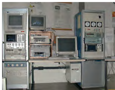
Figure 1-40: The AMA control room.
