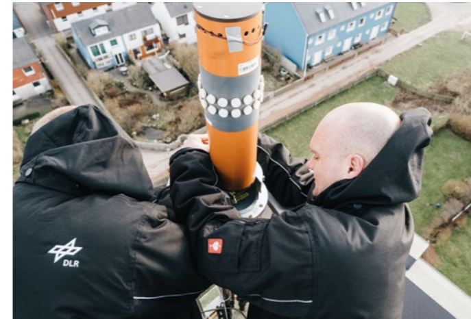
Germany's bright lighthouse is the site for the signal transmission between ship and shore. High above Heligoland, the DLR scientists install their antennas.
