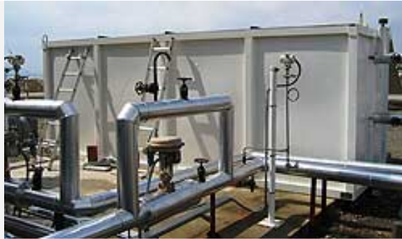
Latent heat accumulator in Almería
