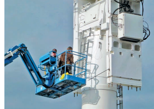
Using the working platform to get to the equipment room of the dish installation – working at a height of 15 metres in occasionally strong gusts of wind.
