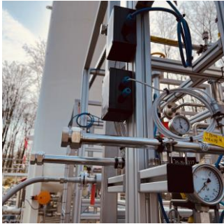
Hydrogen test infrastructure (gaseous and liquid)
