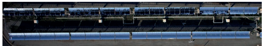
Quadcopter aerial image of a parabolic trough power plant
