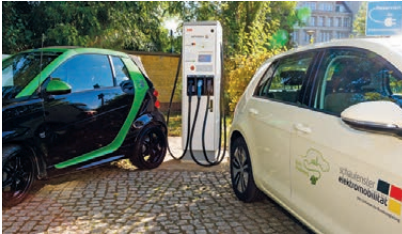
Fast charging station in Berlin
