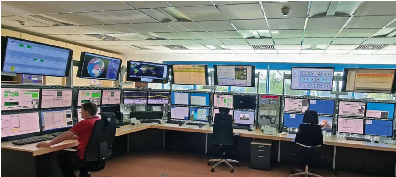
Fig. 4-3 Ground Station antenna control room
