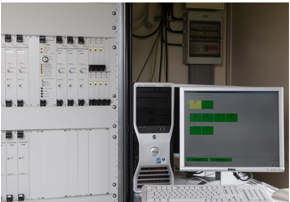
Integrity monitors and equipment at the ground station
