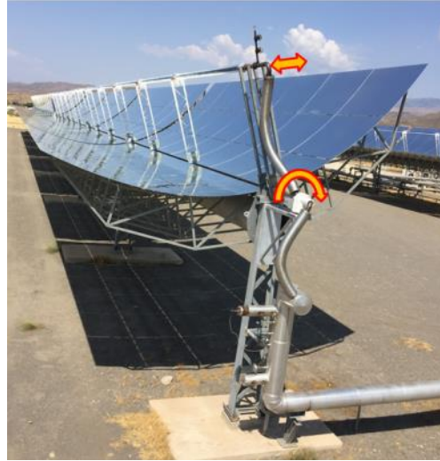
Figure 3. Flexible pipe connectors in parabolic trough collectors accommodate expansion motion (arrow above) and rotational motion (below). Photo: DLR, Plataforma Solar de Almeria owner CIEMAT
